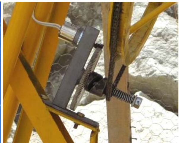
Fig. 9: Motor, gearbox and coupling
